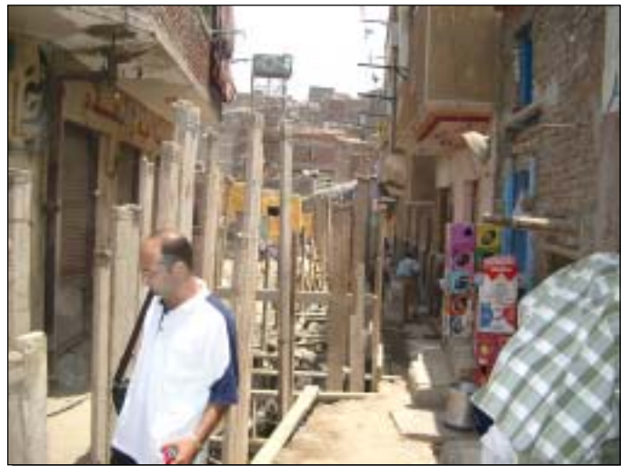
Figure 16: Ongoing activities of the Sewage System
