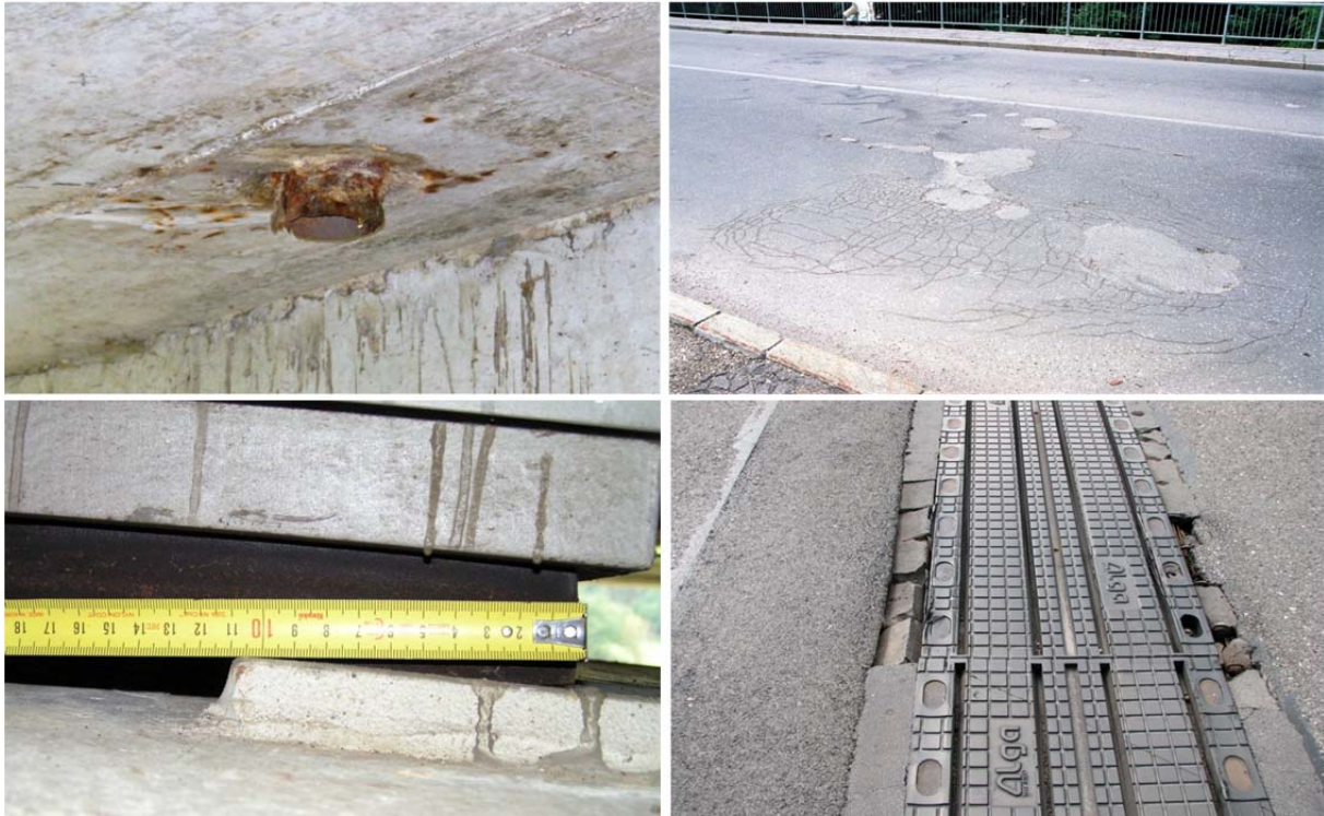
Figure 10 Typical damages that result in costly durability problems on bridges: corroded drainage pipe, damaged pavement and waterproofing membrane, displaced bearing, damaged expansion joint
