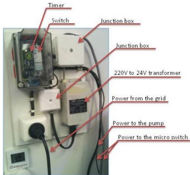
Figure 4 - Electrical system. Photo by author.
