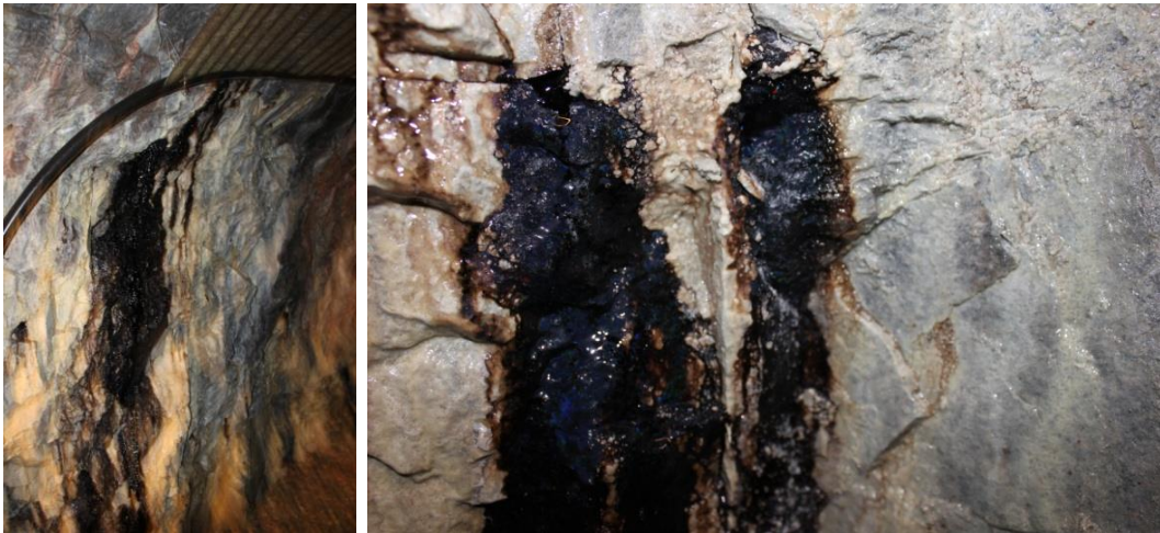
Figure 50 & 51: Black substance leaching from cracks in the mine corridor.
