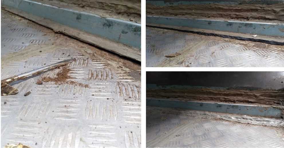
Figure 2: From left to right—cleaning dirt from gap in floorplate, sealing the gap, and applying waterproofing sealant
