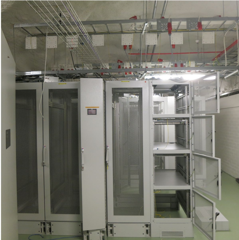
Figure 2. Emptied server racks in HE2.
