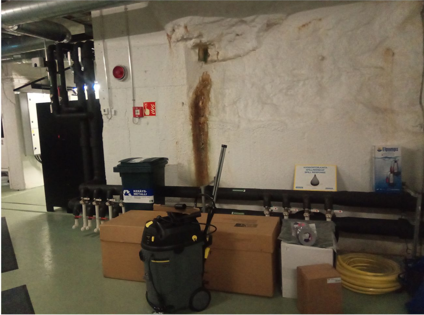
Figure 1. Emptied dataspace, Equinix HE2 data center. Photo: Julia Velkova.
