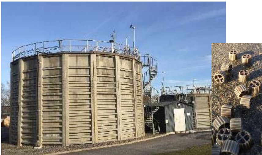
Figure 10. The reject water tank for deammonification at Slottshagens WWTP in Norrköping. The buffer tank can be seen on the right. Insert: Carrier material taken from the tank with biofilm attachment.
