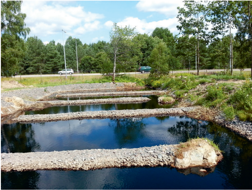
Figure 10. Photograph of the existing vegetative filter immediately after construction in 2013 (and therefore without vegetation).
