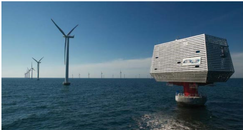
Figure 3: Substation with a 132/33 kV, 180 MVA transformer at Nysted Offshore Wind Farm, Denmark.
