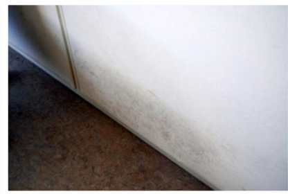
Figure 6 Shoe marks on the wall.
