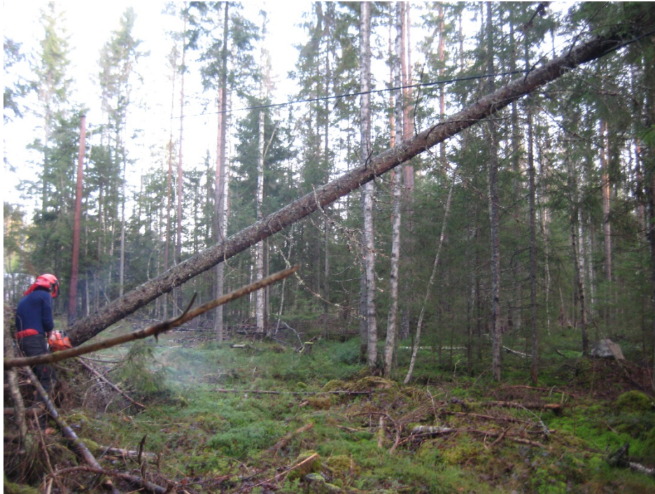
Figure 6: Daniel Heidkamp at Infratek removes a tree from an overhead line. Picture Sabina Stenberg
