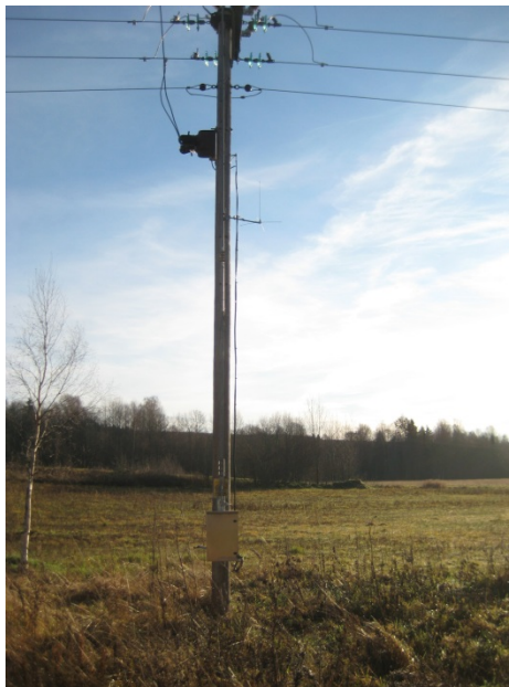
Figure 5: A remote controlled disconnector. The yellow box at the base of the pole is the control equipment. Photo: Sabina Stenberg
