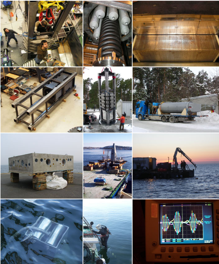
Figure 4.7: Pictures taken from different stages during the construction of the first wave energy converter for the Lysekil wave energy research site.
