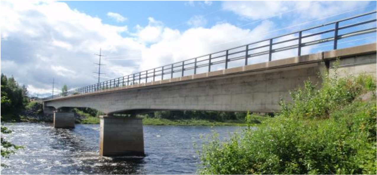
Figure 1. Prestressed Concrete Bridge over Torne River at Autio built in 1963 with three spans and a total length of 134.8 m. View towards SE.
