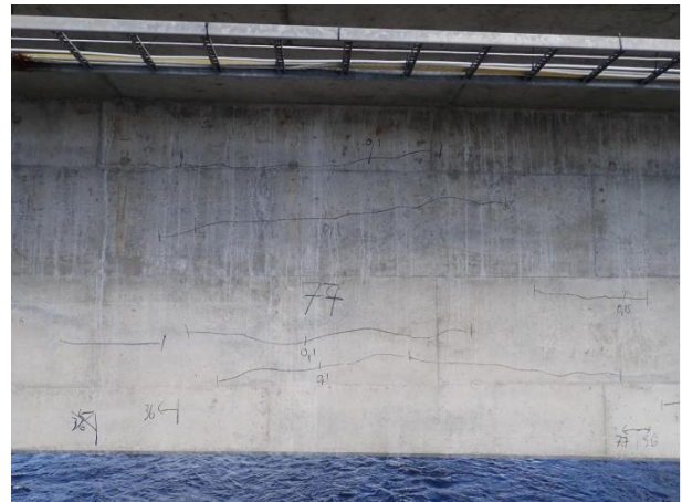
Figure 7. Crack pattern at section 77 in Figure 6 (the 1/4-point) where joints of the prestressing reinforcement are situated. There are five cracks of width 0.1 mm, but they are hard to see for the naked eye.
