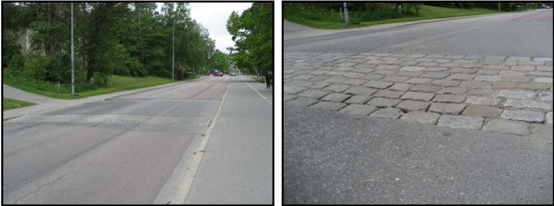
Fig. 4.13 and 4.14. Bump in the middle of the street and photo detail of the bump
