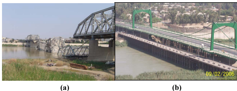
Figure 3: (a) Destroyed parts from Al-Sarafia Bridge have fallen in the river (from www.wikipedia.org ). (b) Temporary bridges parallel to the suspended bridge (from Google Earth).
